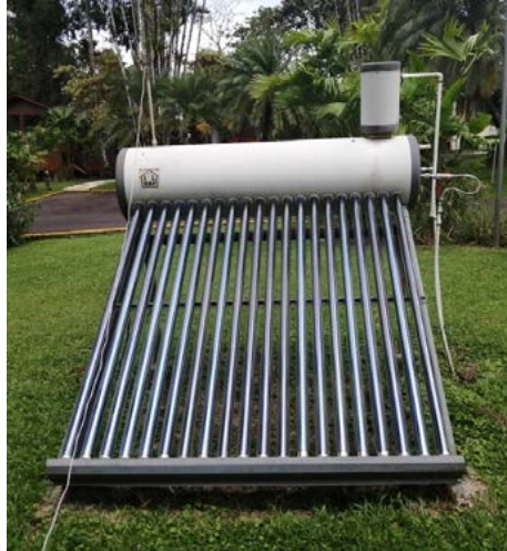
Photo 31: Example of a solar-thermal hot water system, © GIZ, Philipp Denzinger
