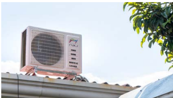
Photo 17: Green AC equipment with R-290 (condenser) © GIZ/Gianfranco Vivi.
