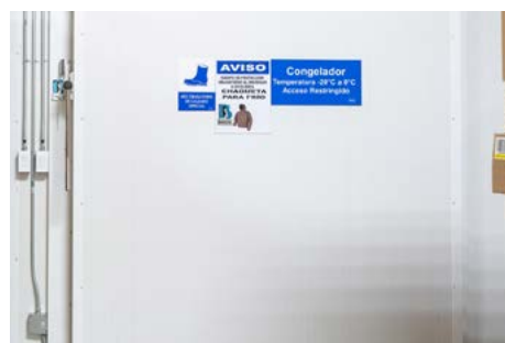
Photo 15: Example of cold rooms with R-290 © GIZ/ Gianfranco Vivi
